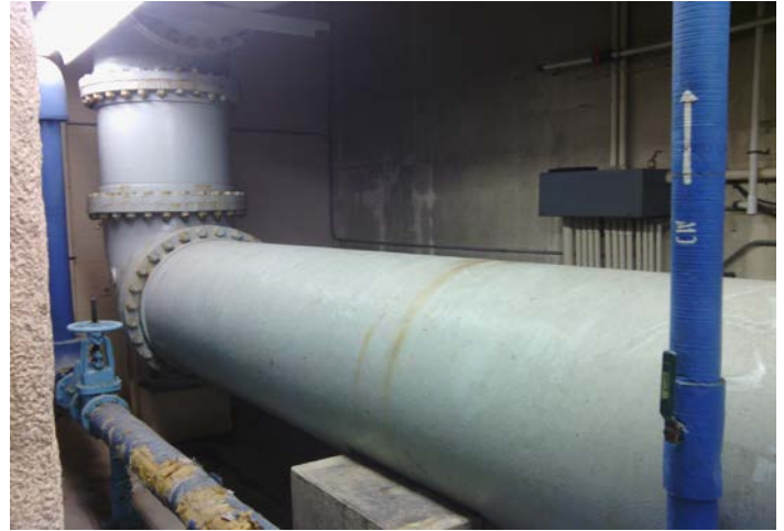
30 inch ductile iron force main
