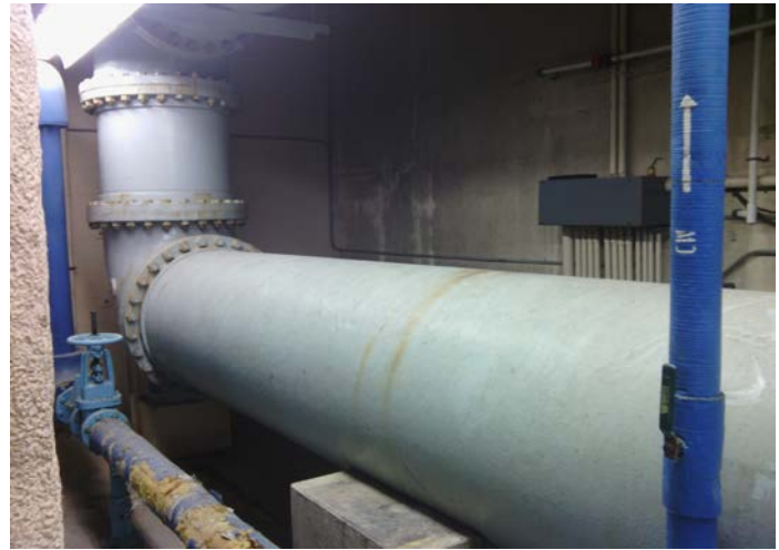
30 inch ductile iron force main
